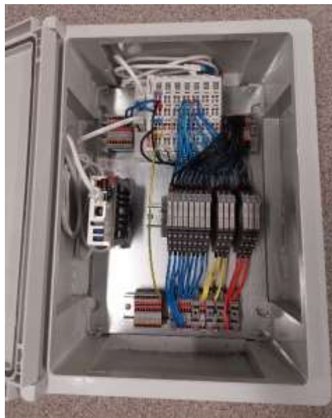
Figure 37: Assembled PLC Junction box
